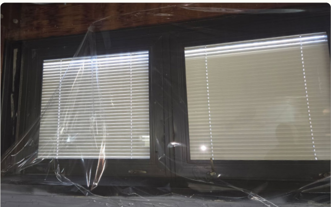
SYSTEMIC BARRIER SCHWARTZ MEN’S SHELTER (City-Owned) Old windows let in water and cold air. DHS instructed VOA-GNY to use temporary shrink-wrap coverings for insulation while our request for funding to replace windows remained pending for months. As a result, windows cannot be opened for temperature control and fresh air, natural light is blocked by the blinds, and the covers contribute to the overall institutional feel of the building.
